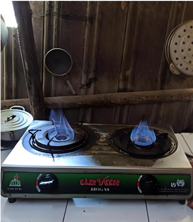
Biogas plant in Huong An, Hue City, Vietnam.
