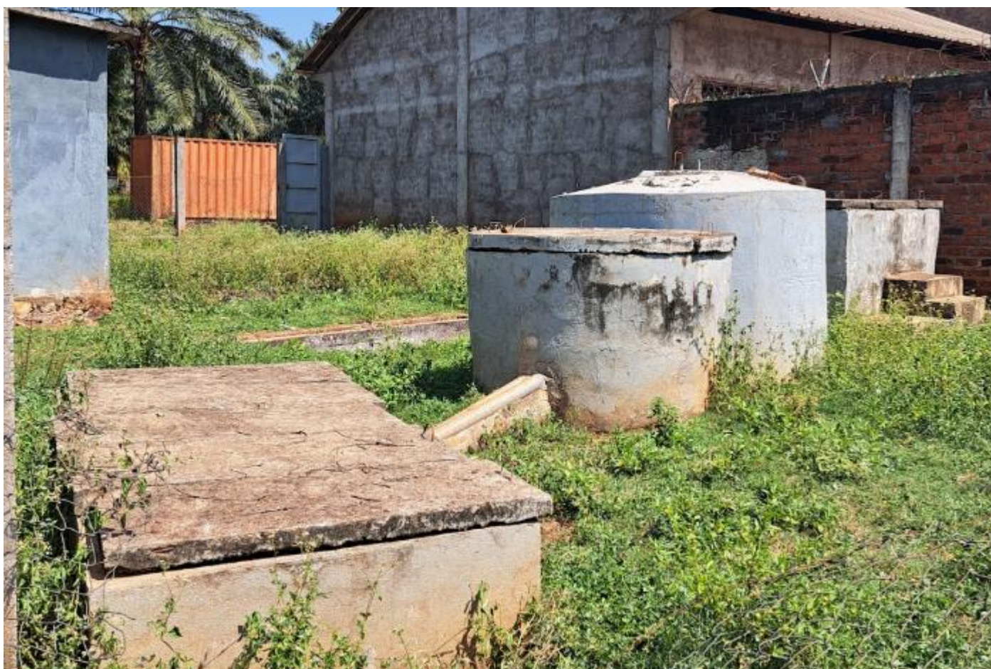
Figure 7. Abandoned, never functioning biogas plant constructed by FAO programme
